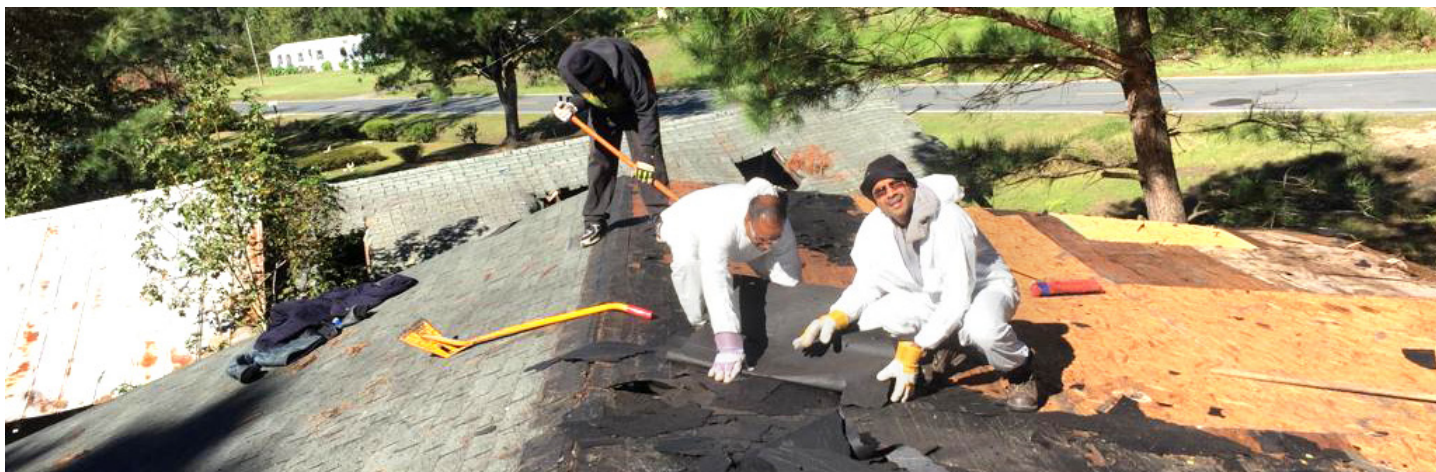
Sewa volunteers Praveen Chand, Dasharath Lohar, Prashant Phirke restoring the roof of a home in St.Pauls
